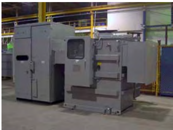
2500kVA Small Power Transformer c/w 15kV Switchgear
