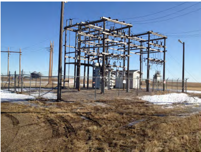
5MVA 72kV Old Wood Pole Substation
